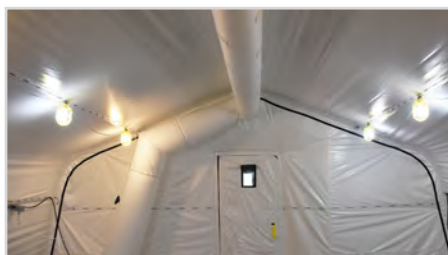
Plenum, lighting, and power receptacles
